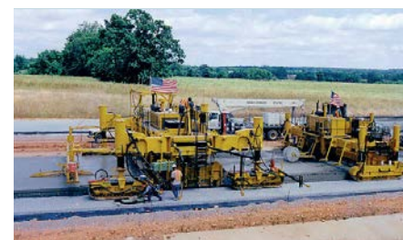
Captions Opposite top: SF-3 with auger. Opposite bottom: SF-6 with a S6 paving kit paving multiple lanes. Top left: SF-3 with super-smoother. Top right: SF-6 paving an interstate. Above: SF-6 working as part of a paving train.
